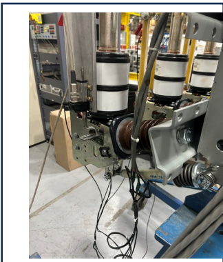
Fig 3. Breaker being Tested (Rear of Breaker)
